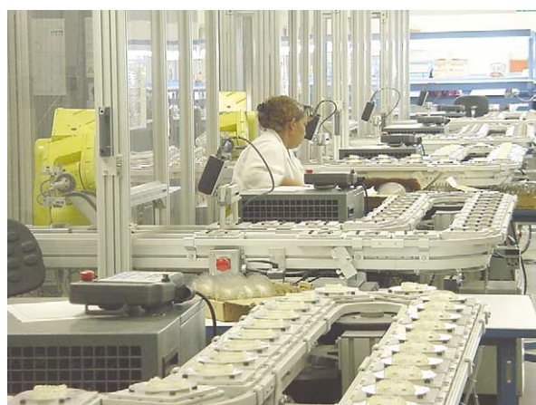
Fig 5. Conveyor to robot (yellow).
